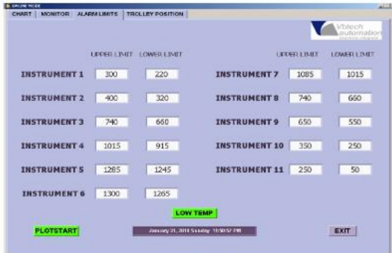
Fig. 7 Alarm limit setting
